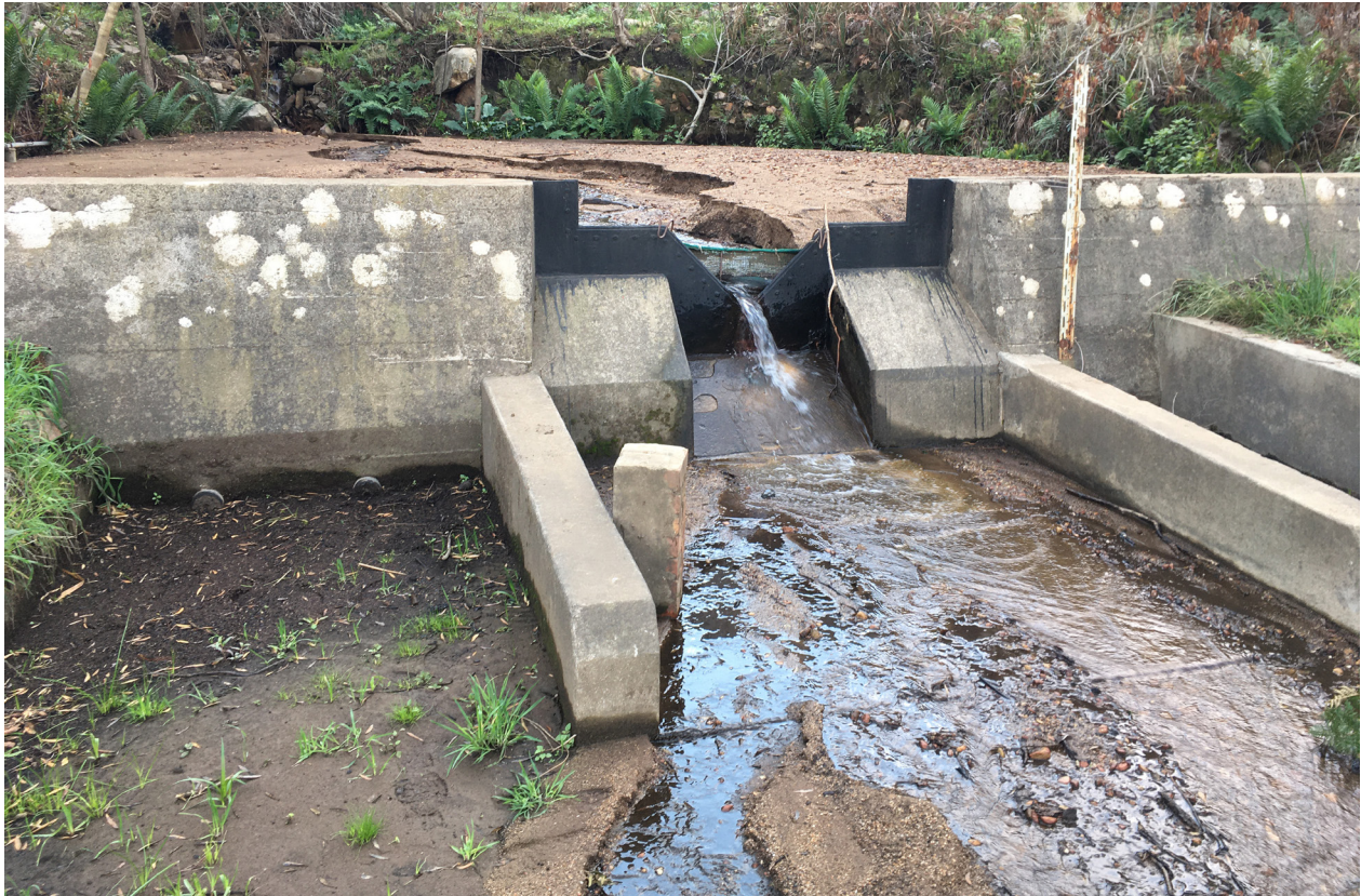
Sediment clogs streamflow measurement weir in Jonkershoek plantation after the 2021 fire.
